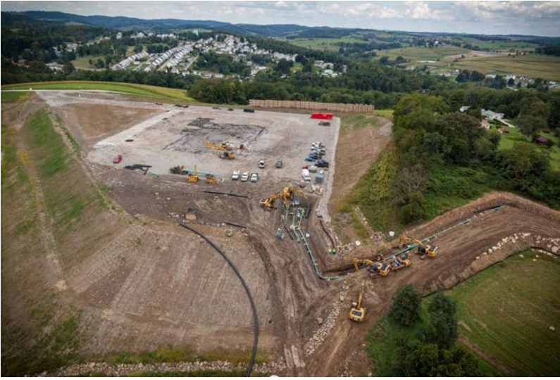
Drilling pad and pipeline construction, Marcellus Shale, Western PA. Rock lined ditches and filter sock around the perimeter contain any water and soil runoff from the site.
